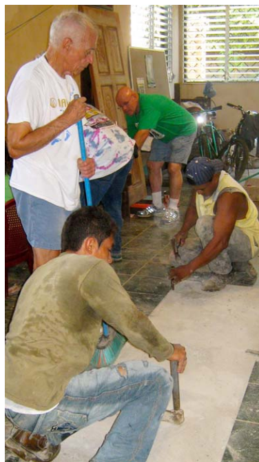
VIM members John Colbert and Mike Sheehan help local workers lay tile flooring.
